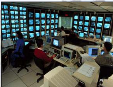
Minnesota DOT's Traffic Management Center
